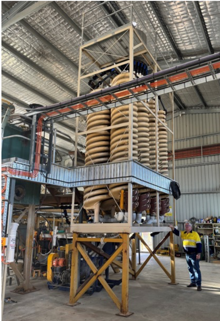
Spiral gold separators will transition Challenger to continuous processing from the previous batch process.
